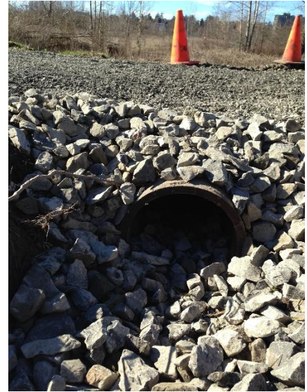
Figure 8: 2in rock material was used at the entrances of the pipe to make it flush with the ground, prevent erosion and improve safety for UBNA walkers.
